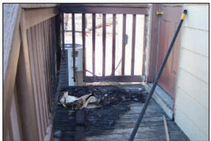
This photo shows damage to a wooden deck from embers.
