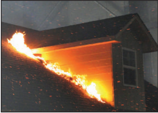
Debris can build up in corners, providing fuel for embers. Photo by Institute for Business and Home Safety Research Center.
